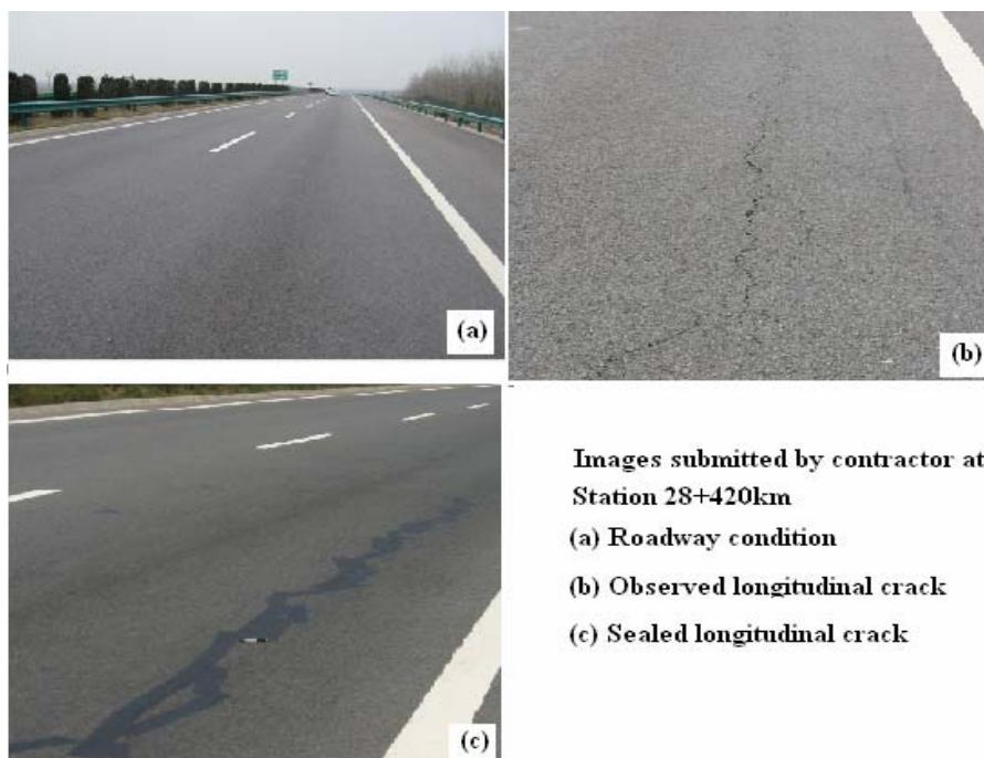
Fig. 4. Reporting and tracking a longitudinal crack using the web-based Chuning PMS.
