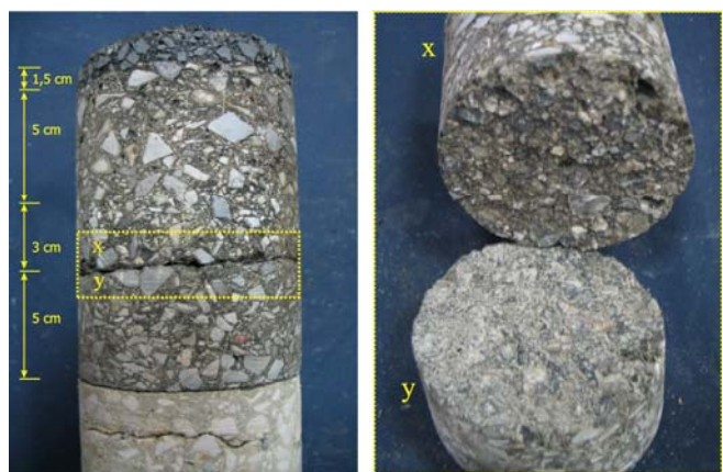
Fig. 8. Core 3b – No Bonding in the Binding Layer, Fully Exposed Aggregate Grains at Connection Surfaces (Asphalt Binder).
