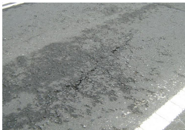
Fig. 2. Top-down Cracking Associated with Segregation
