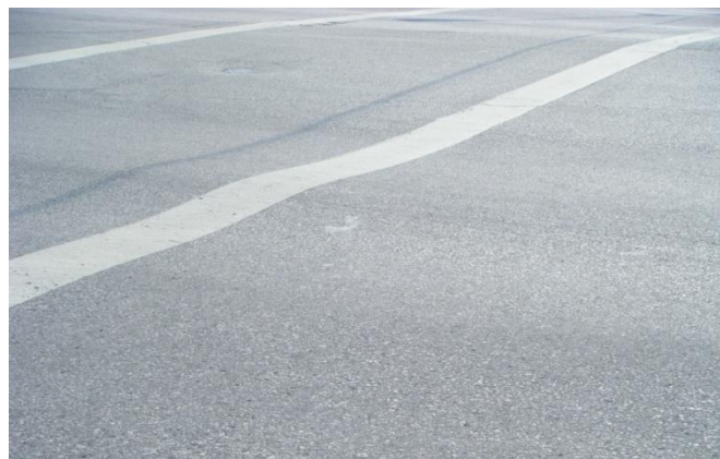
Fig. 1. Pavement with Severe Instability Rutting.
