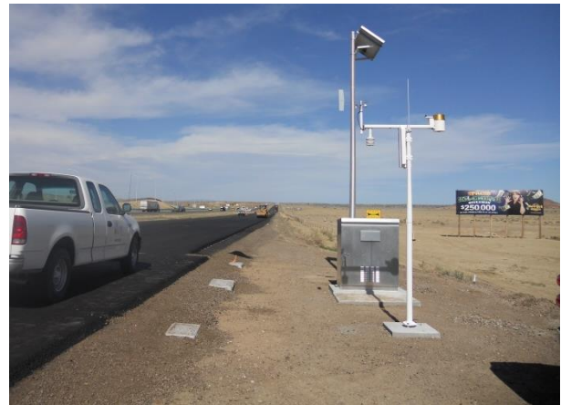
Fig. 2. Installed Weather Station.
