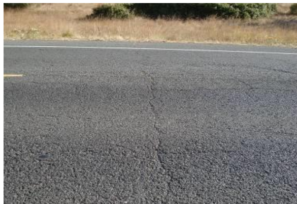
Fig. 1. Existing Pavement Showing Cracking and Raveling.
