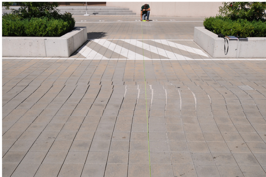
Fig. 1. Damage in a paving block structure because of too little horizontal loading resistance.
